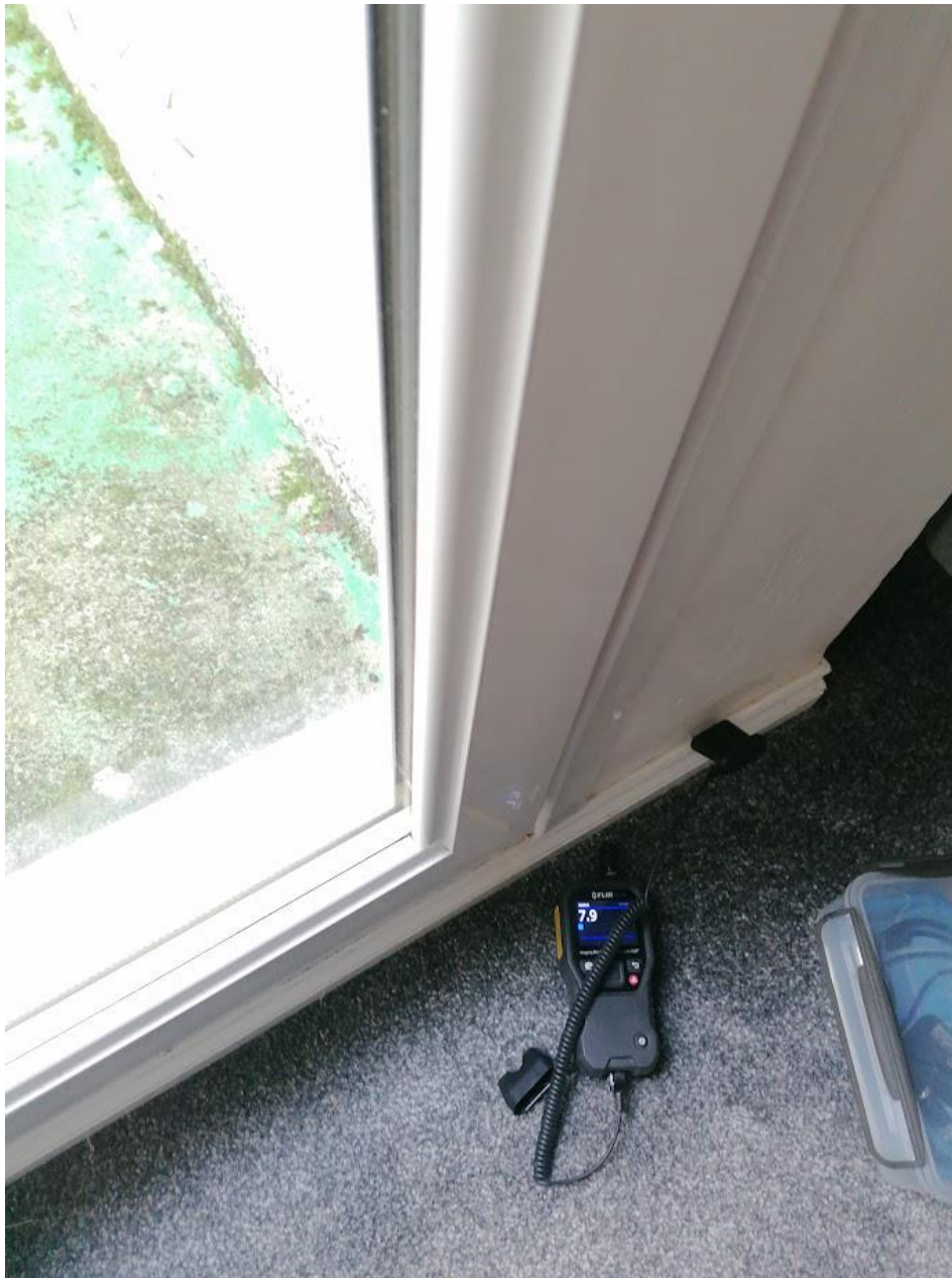
Condensation within the studded wall frame. Please see attached notes to help with humidity on cold wall surfaces.
